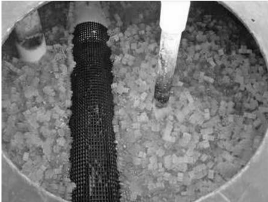
Figure 8. Media and discharge manifold in a MBBR (from Ebeling and Timmons, 2012).
