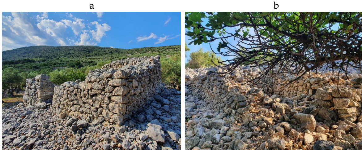
Figure 91. The common current state of many field huts: a) Roof collapsing as the first stage of degradation. b) In an advanced stage of degradation, one of the last indicators of its use is the interior niche (2020)
