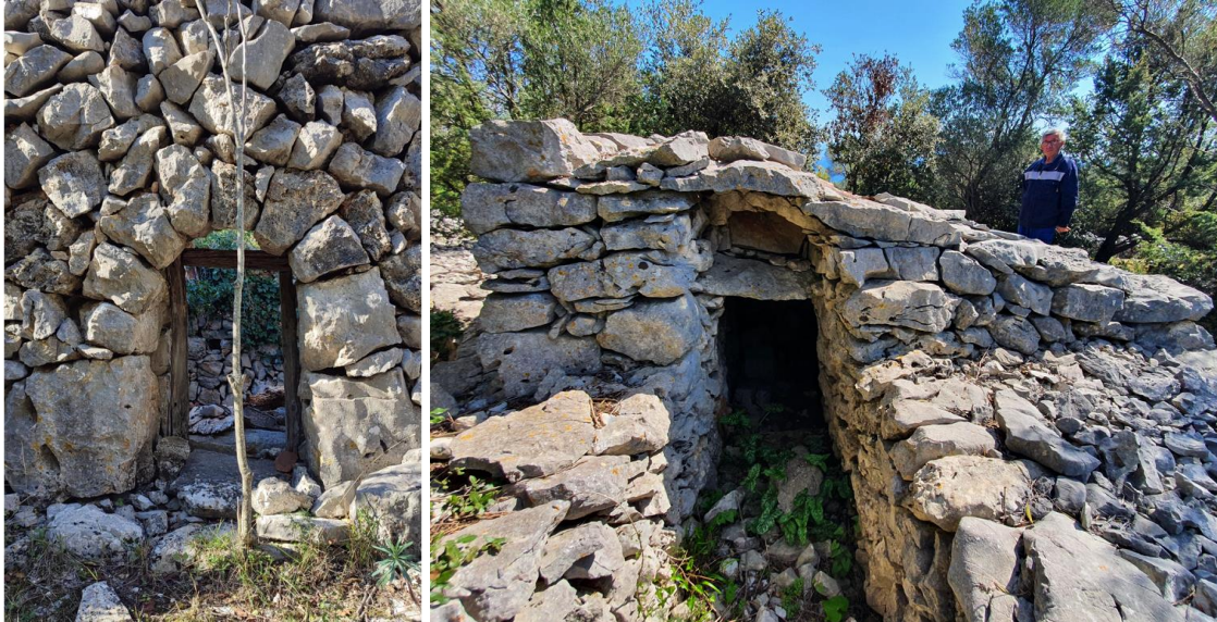
Figure 89. Dry stone livestock sheds and their dry stone constructive elements: a) an arch on the entranceway to a livestock shed, close to Lubenice (2021), and b) a livestock shed close to Arcić (Lovreški), with double lintel (2021)
